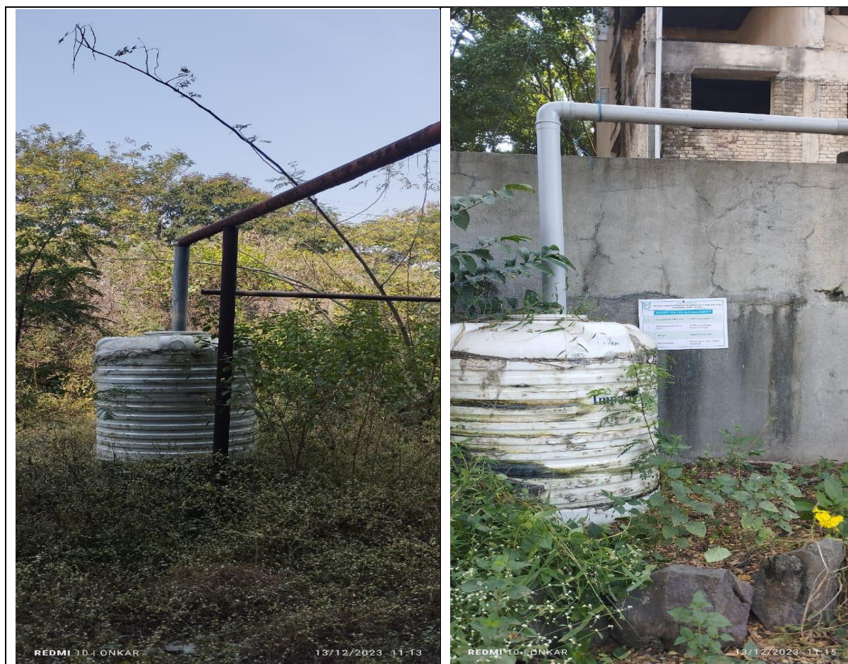
Liquid waste management (water recycling tanks)
