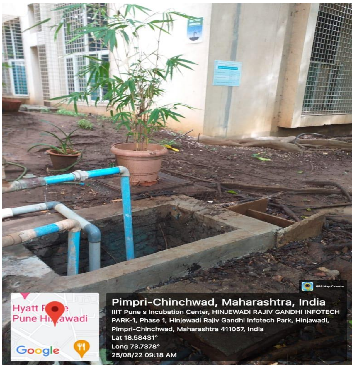
Rain water harvesting
