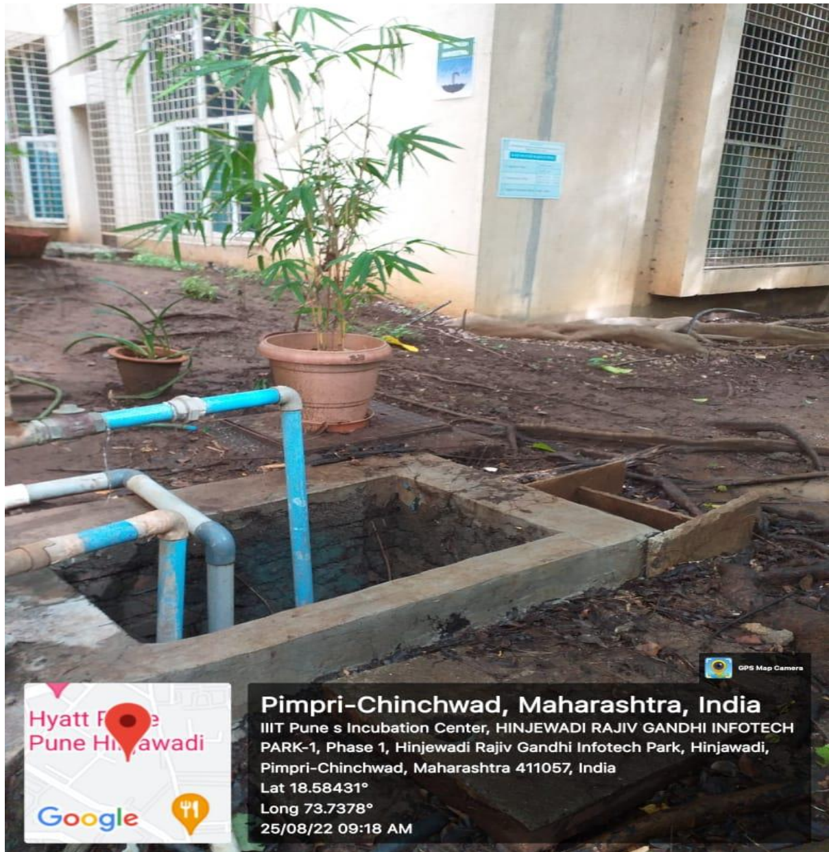
Rain water harvesting plant
